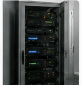
NVR / Control Room
