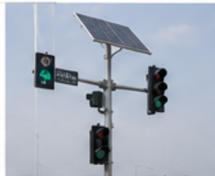
Solar Traffic System
