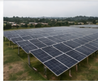
Ground Mounted System
